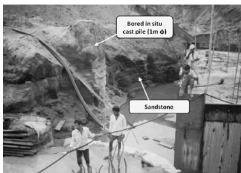
Figure 05: Deep bored pile founded and rock socketted in bedrock for 23 storey structure.
